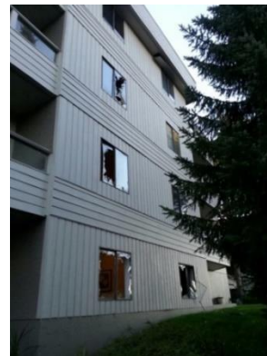
d. Broken windows on the apartment block
