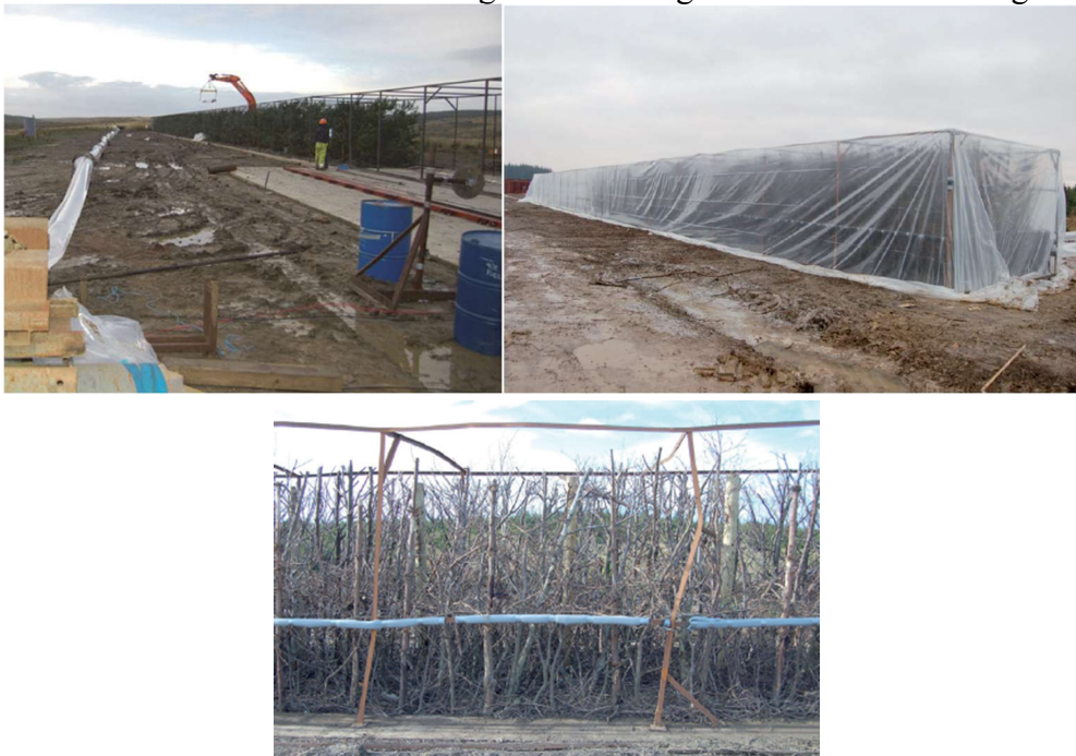
Fig. 10. Tarpaulin-covered metal structure and example of congestion
