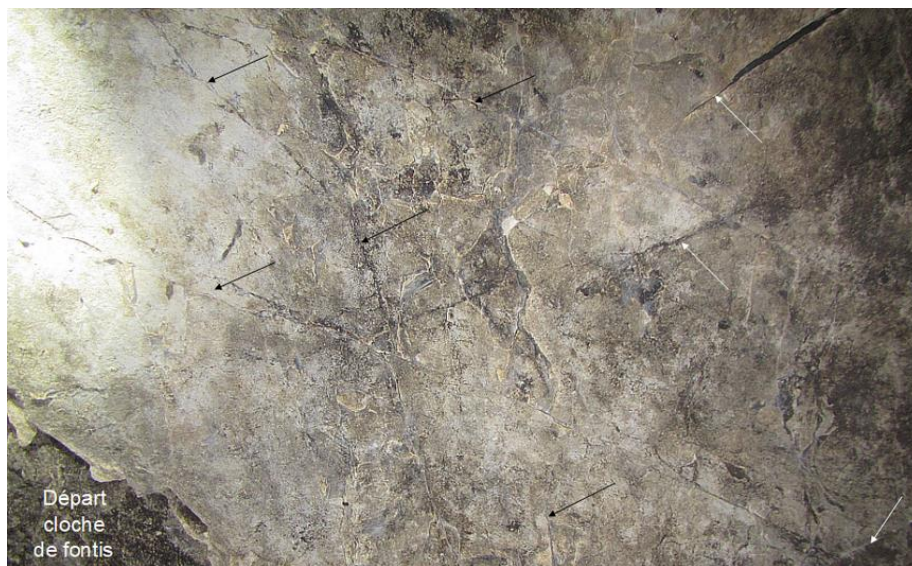
Figure 13. Photos of the roof of one of the galleries. The multiple conjugate fractures (arrows) testify to the intense fracturing of the galleries (Cerema, 2020).
