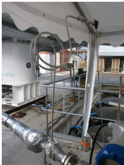
Fig. 6. Picture of the pressure transducer upstream of the flowmeter
