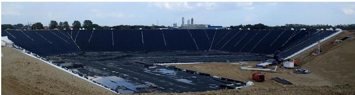
Photo 1. Excavation of the underground thermal energy storage pit in Vojens, Denmark ( http://stateofgreen.com/en/profiles/ramboll/solutions/world-largest-thermal-pit-storage-in-vojens )
