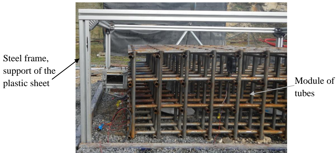
Figure 16 : steel frame which supports the plastic sheet, covering the module of tubes
