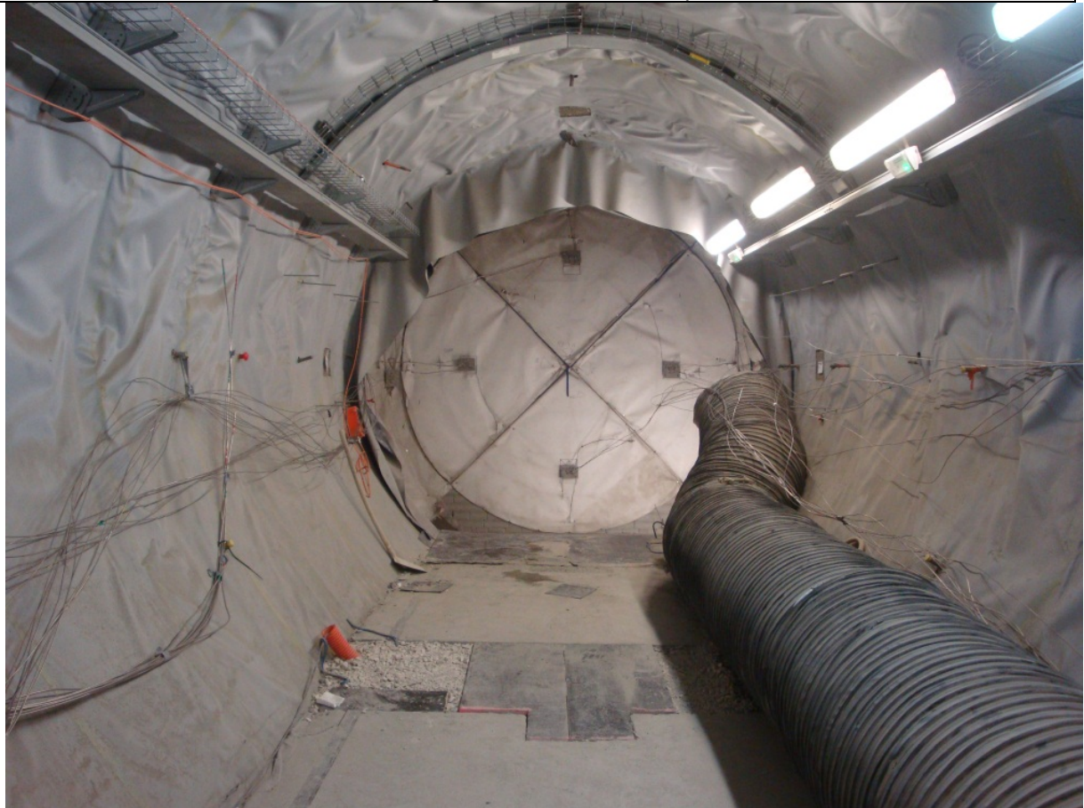
View of the hydration membrane at the interface with the concrete plug (see figure 2)
