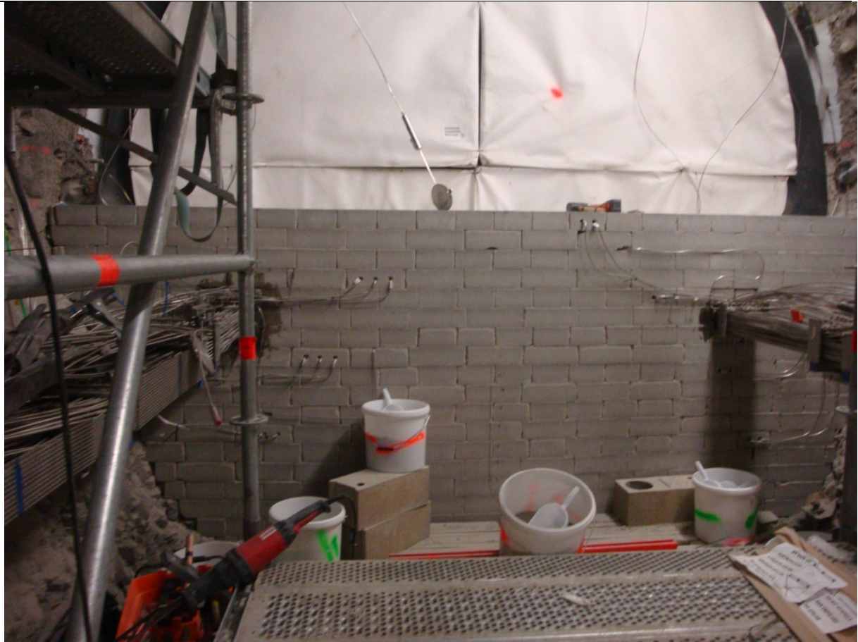
Construction of the seal wall. In the background, we can see an hydration membrane.
