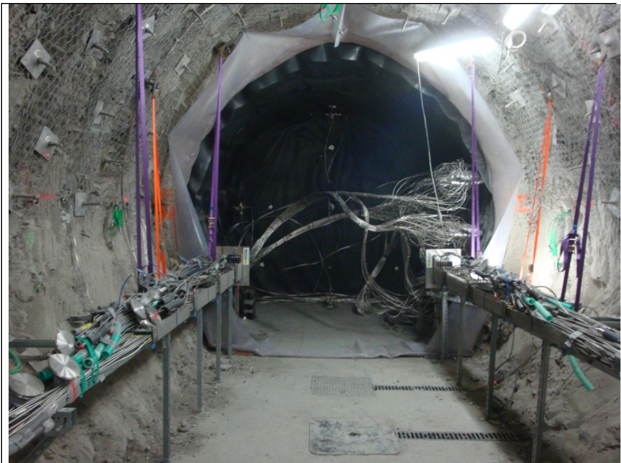
View of the injection chamber before pouring with all the tubing passing through instrumentation boreholes. All the sensors are grouped before the construction of the seal
