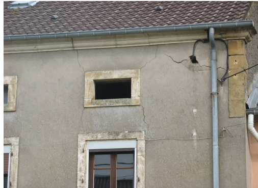
Figure 4. Example of limited damage incurred following the subsidence in Rochonvillers (Roc_2008)
