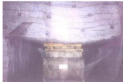
Figure 5: Example of separation of roof (source, MDP A 2015).
