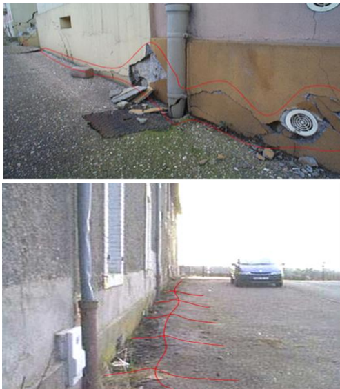
Figure 3. Example of serious structure damages due to subsidence – Iron mine – Lorraine – France.
