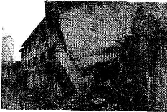
Fig. 2: Building collapse due to insufficient reinforcement.
