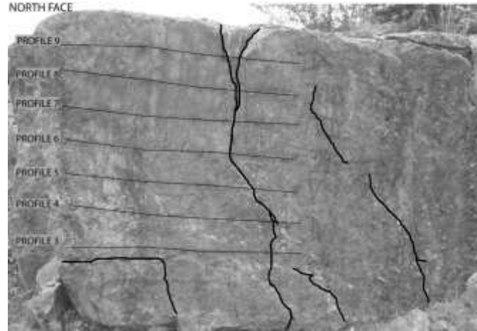
Figure 18: Depict of the North Face of the block in Chambéry (73). The black lines reveal the different discontinuities observed. The black horizontal lines identified each radar profile, profile 3 to 9 from the bottom to the top.
