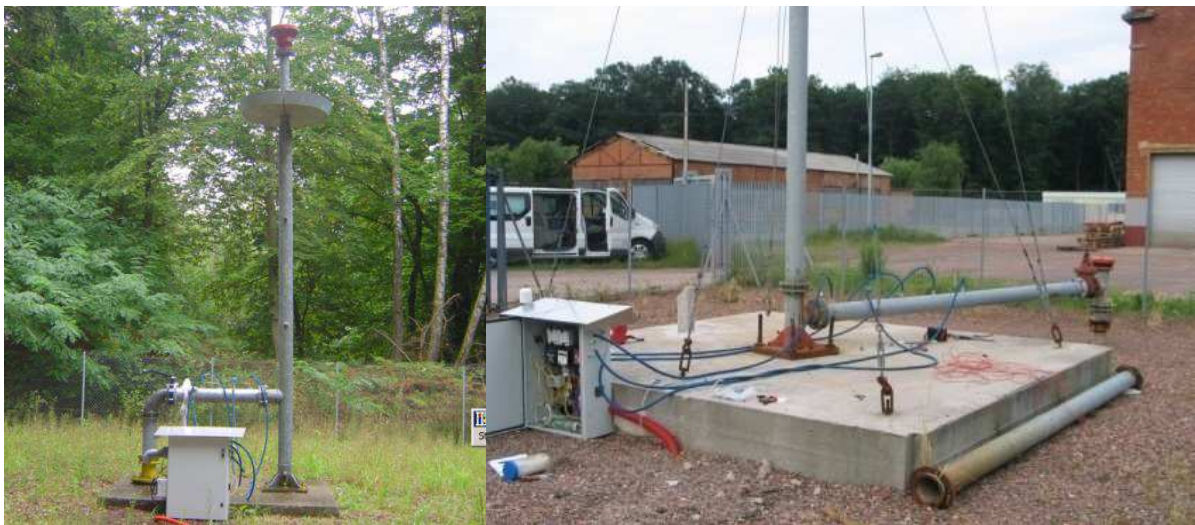
Figure 1: Photographs of the vent SDEC OUEST 1 (left) and BARROIS shaft with a vent (right).
