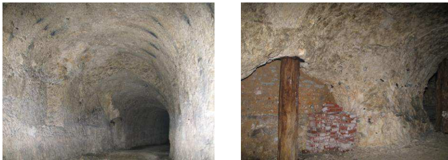
Figure 4: Some views of a remaining chalk mines in Lorroy, close to the one collapsed in 1910.
