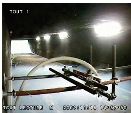
Figure 9: Observation of a gas layer in the lower part of the tunnel.
