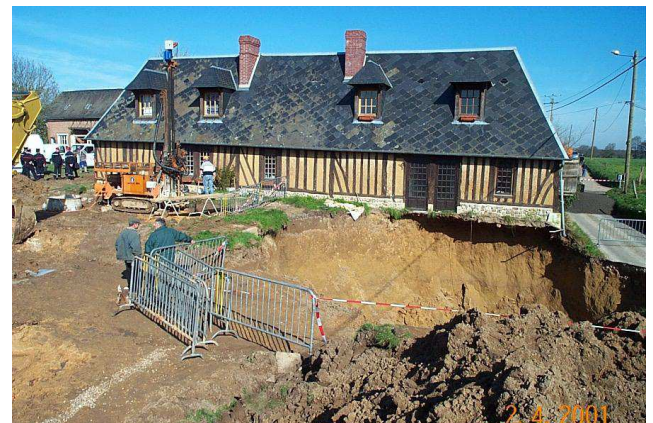
Figure 2: Sinkhole having caused a fatality within a French urban area (source CETE/MEEDDAT)..
