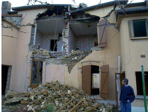
Figure 2. Damages generated by the Auboué subsidence event.
