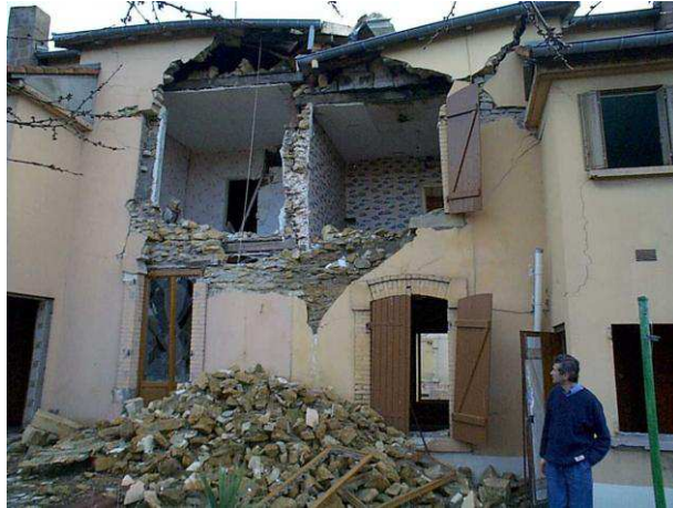
Figure 2. Damages generated by the Auboué subsidence event.
